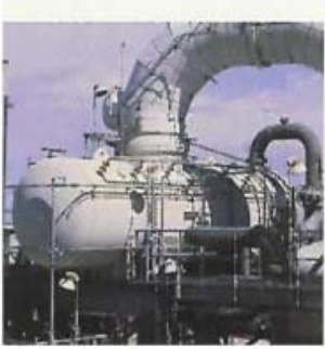
Process vacuum condensers
